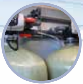
Ion exchange units for water softening
