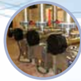
UV units work to reduce chlorine and ozone usage
